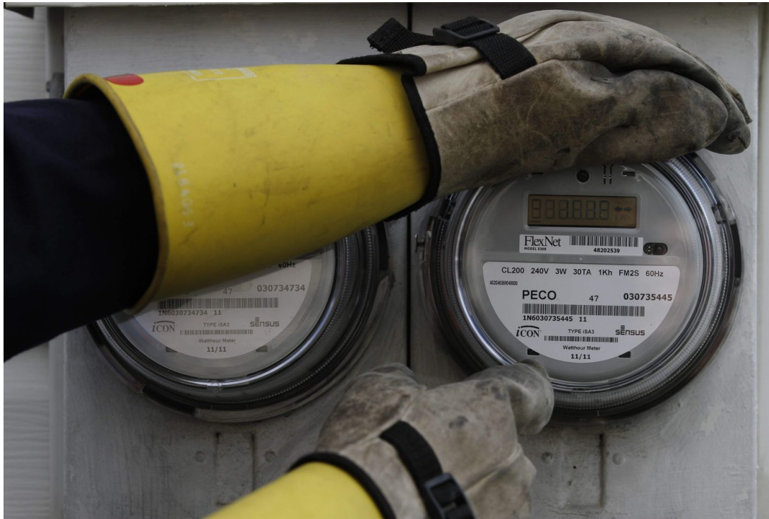
A Peco worker installs an electric meter. MICHAEL S. WIRTZ / File Photograph
