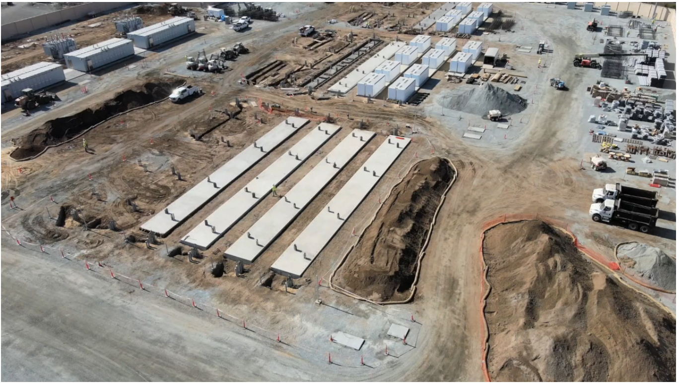
The Moss Landing battery storage project under construction near Monterey, California in October. VIDEO COURTESY OF EKM METERING
