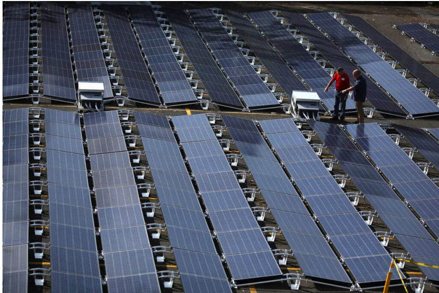
Solar panels being installed at the San Juan Children’s Hospital in Puerto Rico. Alvin Baez/Reuters
